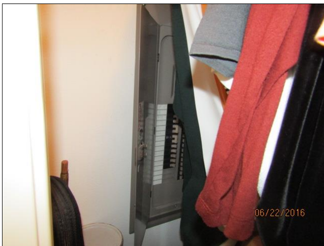
A. Item 1(Picture) Service Panel in Closet at northeast bedroom.
