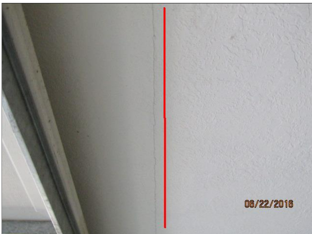
F. Item 2(Picture) Drywall crack in garage indicated the left of red line in photo
