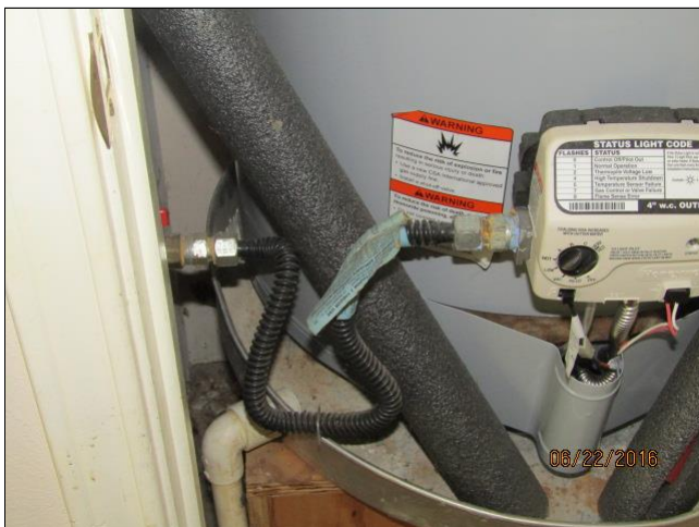
C. Item 3(Picture) Flexible gas Connection Line at Water Heater.
