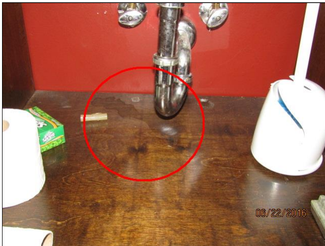
B. Item 1(Picture) Water stain in Half Bath.
