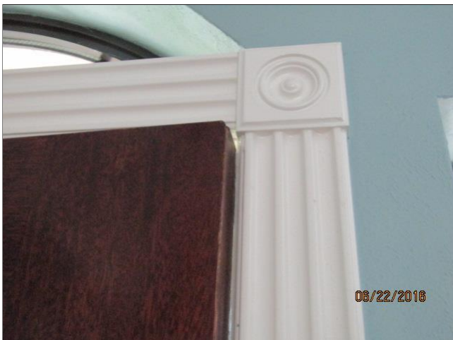
G. Item 1(Picture) Entry Door sticking at door frame
