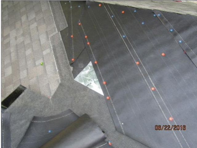
C. Item 2(Picture) Sufficient use of Valley metal flashing.
