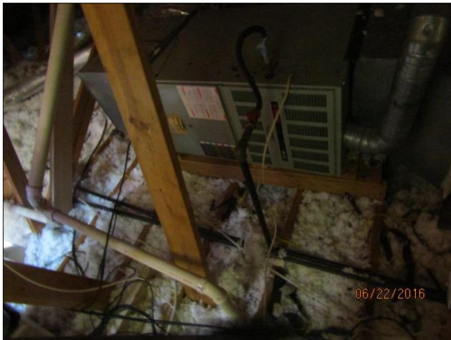
A. Item 1(Picture) Missing Secure work platform at front of Furnace about Garage.
