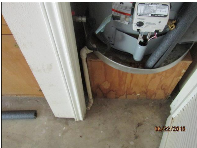
C. Item 2(Picture) Water Heater Drain Pan/ Line
