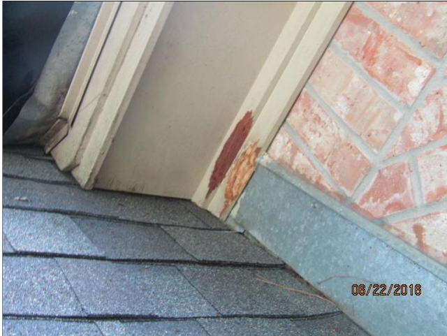
E. Item 1(Picture) Damage at Front Gable roof Freeze Board
