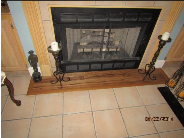
J. Item 1(Picture) Combustibles should not be used as Hearth Extension.
