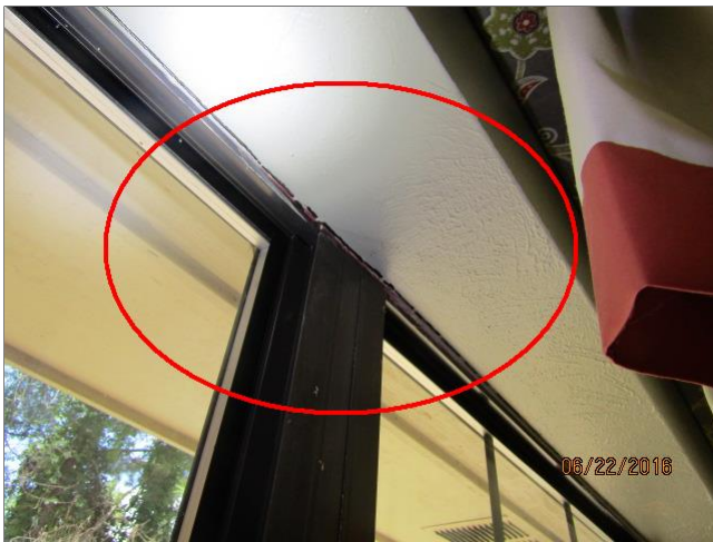
H. Item 2(Picture) Failing sealant at window head in den.
