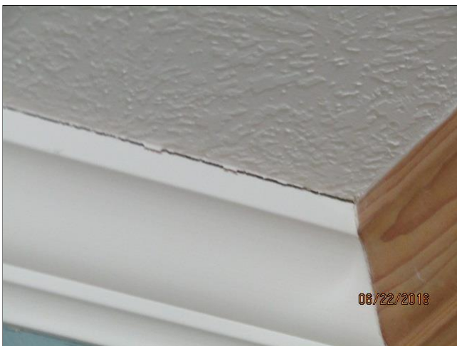
F. Item 3(Picture) Cosmetic failing sealant at ceiling in office.
