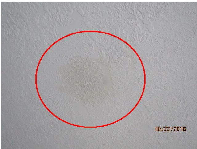
F. Item 1(Picture) Ceiling Drywall stain In Garage.
