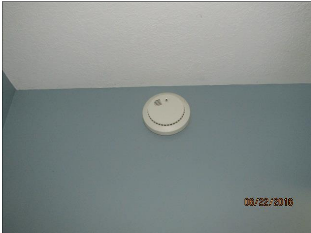
B. Item 1(Picture) Inoperative Smoke detectors throughout home.
