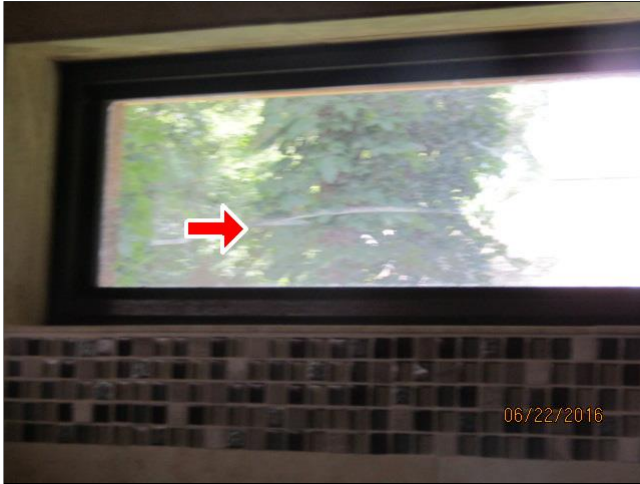
H. Item 1(Picture) Crack in Glazing.
