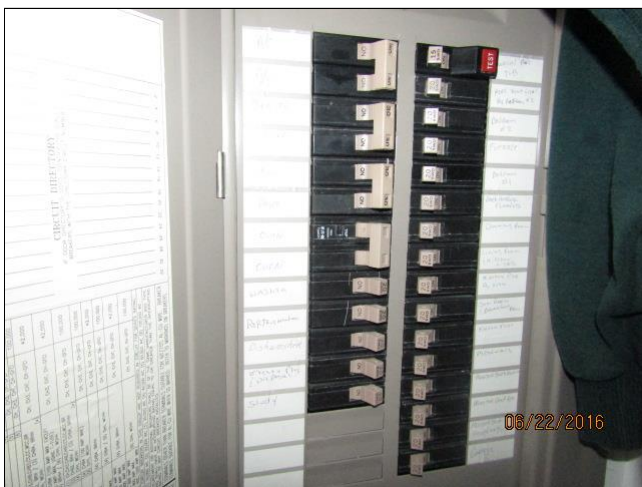
B. Item 2(Picture) Branch Circuits Labeled.
